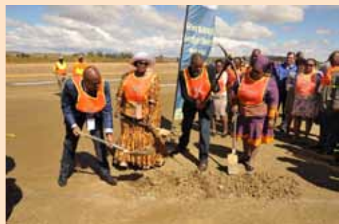
Dihlabeng Local Municipality Mayor Tjhetane Mofokeng, Cooperative Governance and Traditional Affairs and Human Settlements MEC Ollly Mlamleli, Premier Ace Magashule and Social Development MEC Sisi Ntombela turning sods to officially launch the Bulk Water Service Project in Paul Roux.
