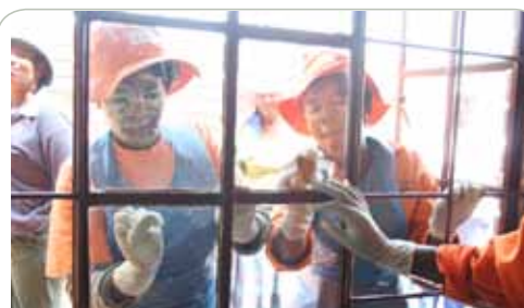
Members of the Zivuseni project cleaning new fitted windows at the Bekkersdal East Clinic.
