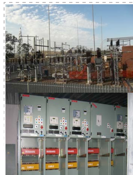
Thornhill electricity substation
