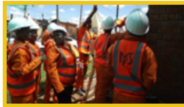
The youth from Matjhabeng Local Municipality doing practical training on installation of decoders.
