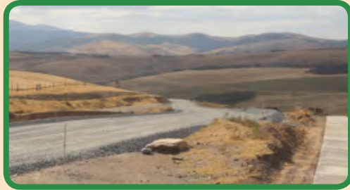
The construction of a tar road from R61 to Nkantolo village is in progress.
