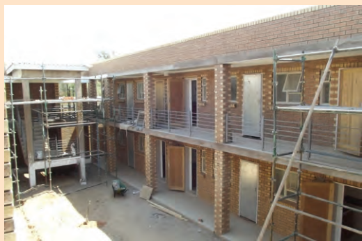
The SAPS single quarters accommodation in Keimoes is nearing completion. It will include two flats for people with disabilities.
