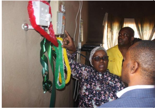
The Minister and Major of Lephalale Switch on electricity at one of the households at Ga Seleka. 732 were switched on.
